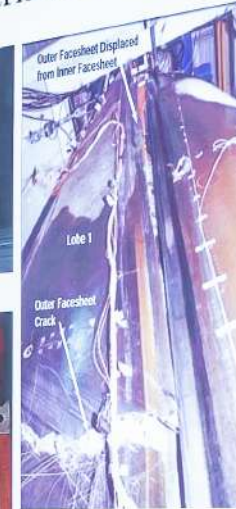
Cryogenic Tank Failure
